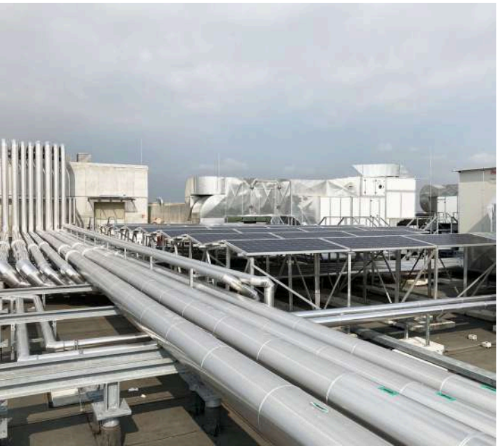
Pannelli fotovoltaici in copertura / Photovoltaic panels on the roof
